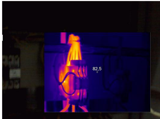
Gambar 2. Hasil scanning thermograph kontaktor panel kapasitor bank IRM
