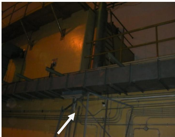
Gambar 2: Exhaust service area
