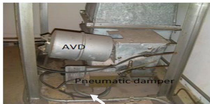
Gambar 7: Damper pada ducting supply udara concrete cell .
