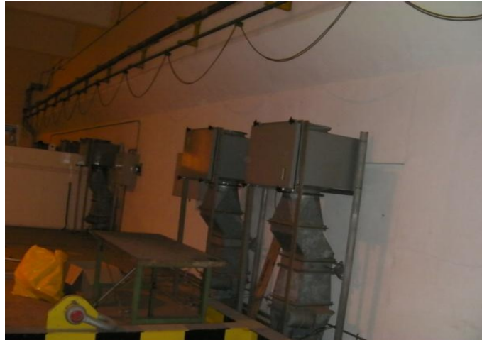
Gambar 3: Filter bank Supply udara hotcell ZG101- ZG103
