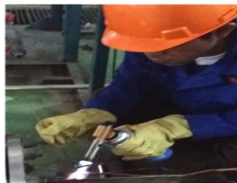
Pematrian pipa evaporator
