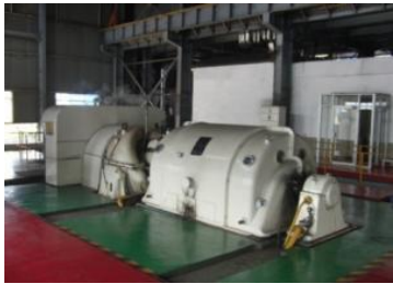
Turbine & Generator Bobot 25 %
