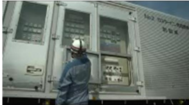
Startup of gas turbine generator car
