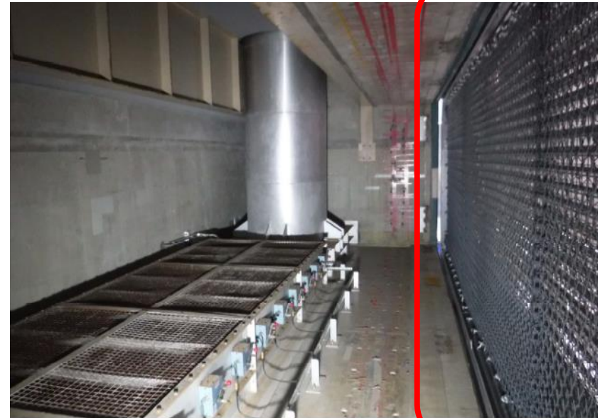
Tornado protection net at louvers
