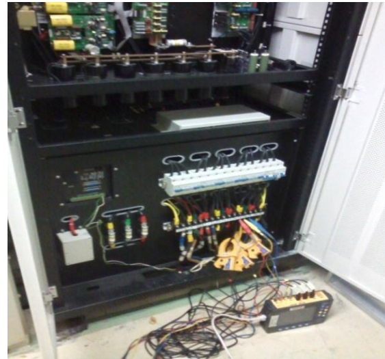
Gambar 4. Pengukuran output inverter BTP03
