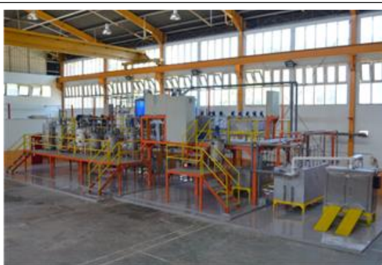
Figure 3: Pilot plant of uranium, thorium, and rare earth elements extraction in BATAN
