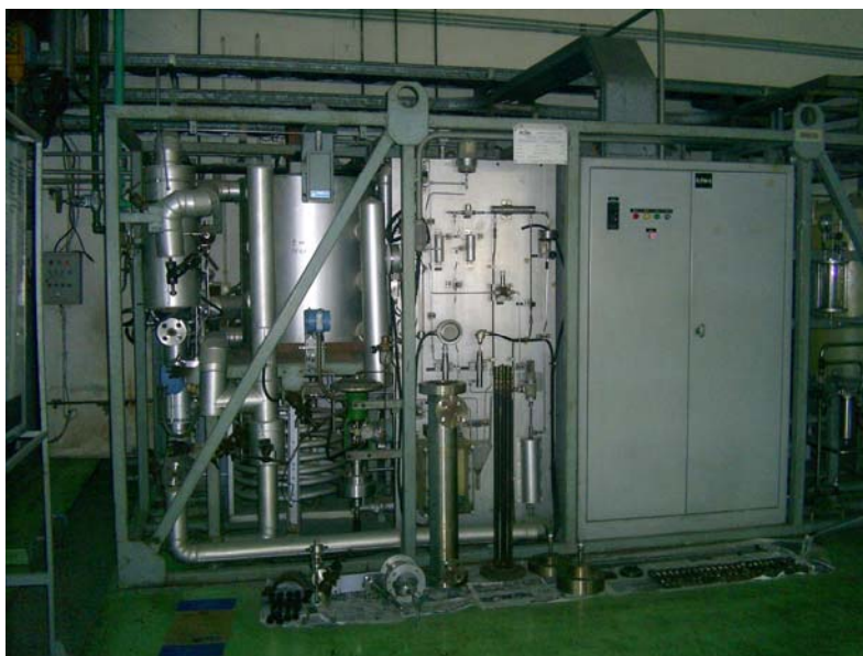
Gambar 1. Untai Uji Korosi ( Primary Loop )
