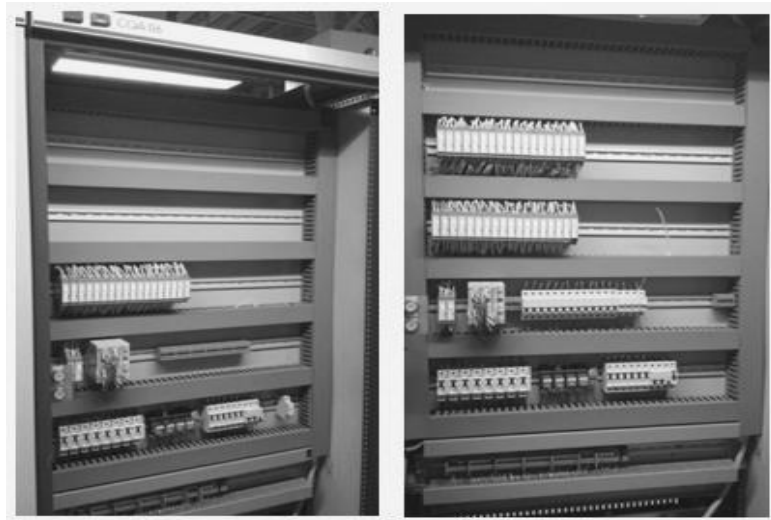
Gambar 7. Instalasi distributor aktif di ruang marshalling kiosk
