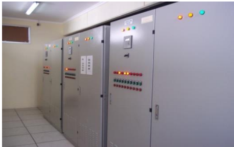
Gambar 2. Panel kapasitor bank BHA/BHB/BHC RSG-GAS sebelum dipasang exhaus fan [1]
