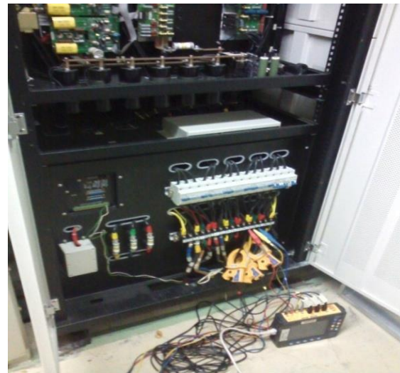
Gambar 4. Pengukuran output inverter BTP03
