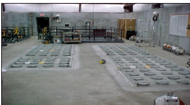
Figure 5. Interim Storage of Radioactive Waste Facility as Downhole.
