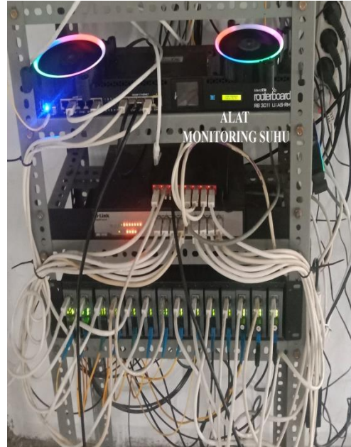
Gambar 9. Prototype dipasang diruang server
