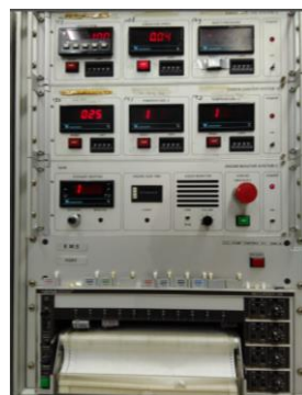
Fig. 2.4.1. Engine Monitoring System (EMS)
