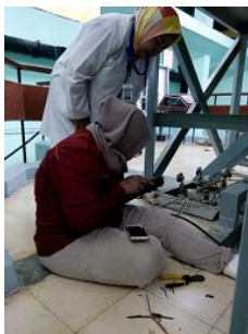
Instalasi suplai daya deck reaktor
